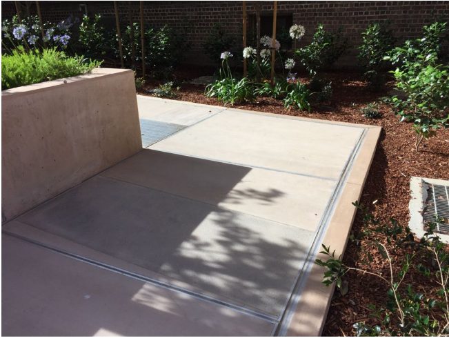
Example showing the joint can be integrated into paver system adjacent to landscaping
