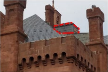
Southeast roof. Existing elevator penthouse to be removed (shown in dashed red lines).
