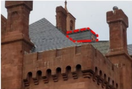
Southeast roof. Existing elevator penthouse to be removed (shown in dashed red lines).
