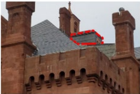
Southeast roof. Existing elevator penthouse to be removed (shown in dashed red lines).
