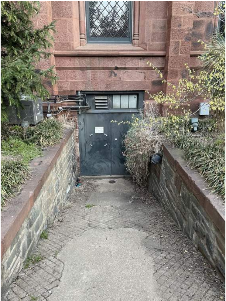
Existing ramp and door at the southeast corner of the Main Building.
