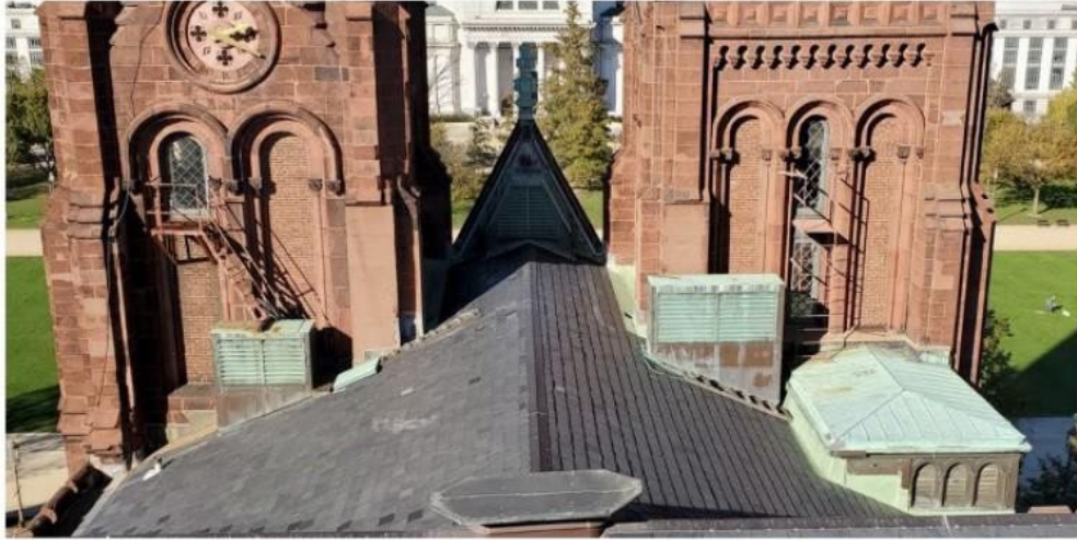
Existing conditions of roof access ladder and stairs at the south elevations of the Flag and North Towers.
