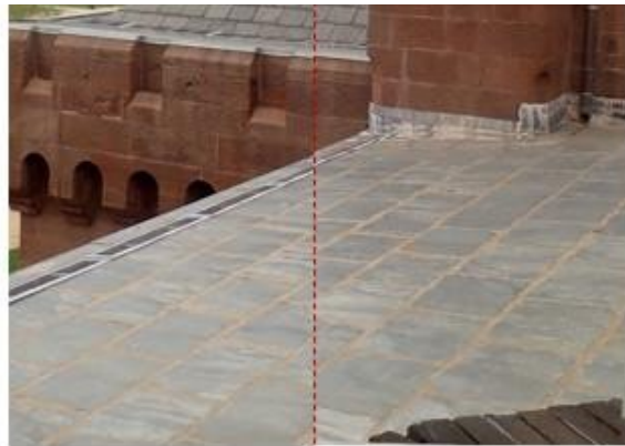
Proposed and existing montage demonstrating the dimensional roof change over the East Range.
