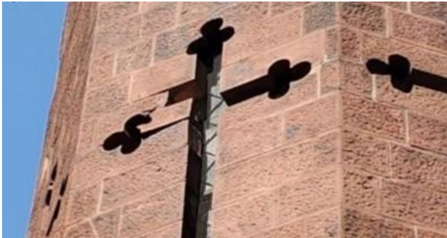
Displaced Seneca sandstone masonry at the Octagon Tower.
