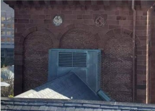
Existing condition of the South Tower peaked roof and mechanical bulkhead to be removed, and the blind arches infilled with brick masonry.
