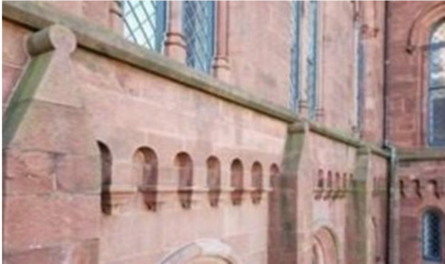
Seneca sandstone with biological growth staining.
