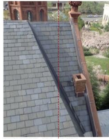
Proposed and existing montage demonstrating the dimensional roof change over the Main Building.
